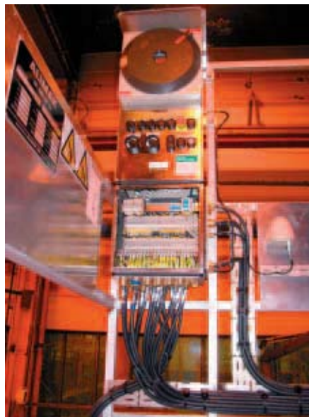
Figure 4: Explosion protected control panel 8125 (with connection chamber open) on the top of the lift car
