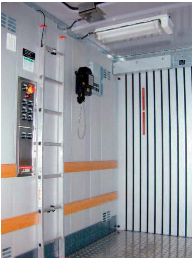
Figure 5: Interior view of the lift cage with explosion protected operating panel 8146, explosion protected emergency light fitting 6008 and explosion protected telephone
