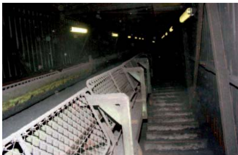
Figure 2: The maintenance catwalks along the coal conveyor belts are illuminated with ECOLUX 6600 lighting fittings
