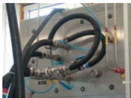
Figure 5: Media supply into the explosion protection compartment
