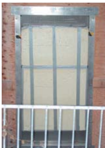
Figure 6: Explosion pressure relief on the explosion protection compartment
