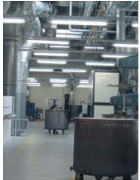
Figure 7: EXLUX 6000 lighting of the production facilities
