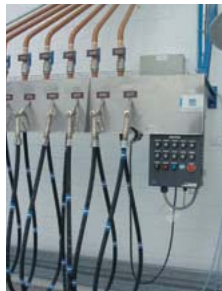
Figure 4: Interior view of distribution panel
