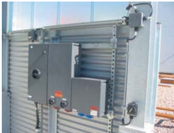
Figure 3: Socket-outlet board in the outdoor raw material-delivery area
