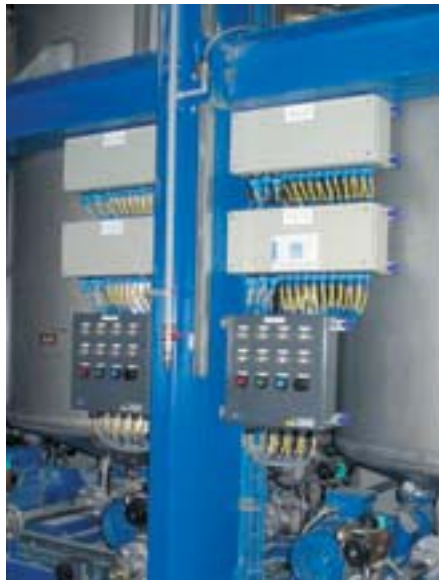
Figure 6: Control switch 8008 and control station 8146 in the intermediate store's filling system
