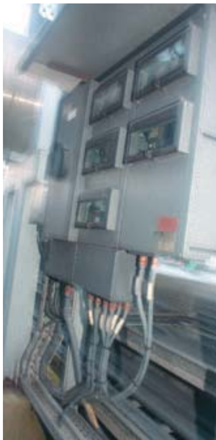
Figure 2: Explosion protected distribution fuse-board at oil offloading stations in the harbour
