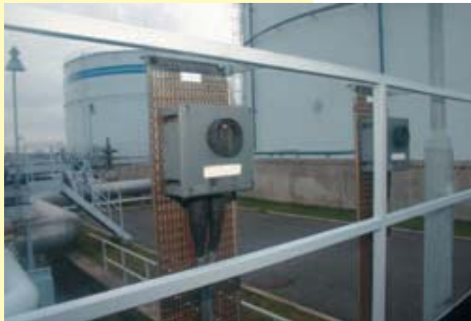
Figure 1: Explosion protected main switch in a tankfarm
