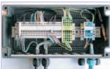
Figure 10: Example of nonconforming equipment (e.g.: open cable glands, direct connecting wire from Ex i to Non Ex i side)
