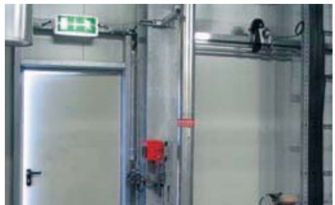
Figure 9: Use of the emergency luminaire 6108 with pictogram, and the horn 8491 and fire detector 8146
