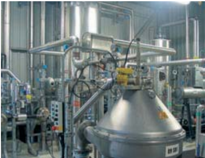
Figure 5: Centrifuges for separation and purification
