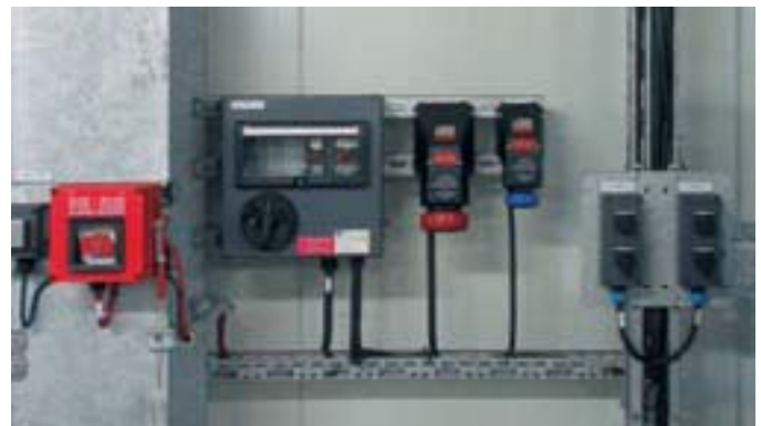
Figure 8: Distribution fuse board 8146 with plug and sockets 8570 and 8571, in addition to control devices 8040
