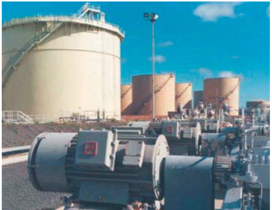
Figure 1: Explosion protected electrical drives in a chemical plant
