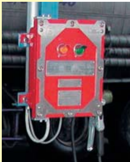
Figure 1: Explosion protected earth monitoring device in a tank filling plant
