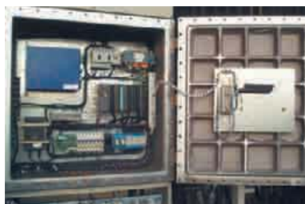
Figure 8: Various locally installed control systems and distribution panels in flameproof enclosure
