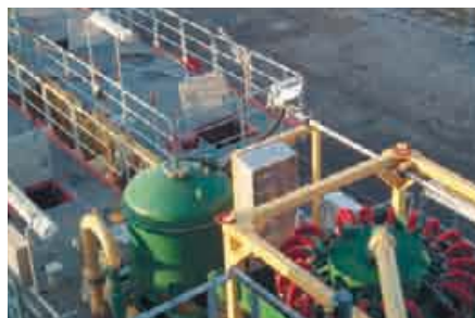
Figure 9: Effective illumination during drilling work with explosion-protected EXLUX 6000 light fittings for Zone 1
