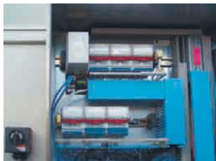
Figure 7: Process automation on the rig is undertaken using 4 Remote I/O systems IS1
