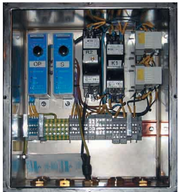
Figure 6: Temperature controllers and safety thermostats. Tranberg delivered temperature controllers for more than 3,000 measuring points
