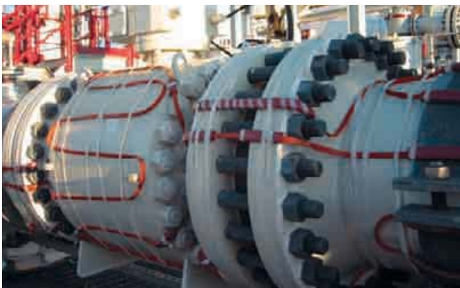
Figure 5: Heated valves before the thermal insulation is mounted. Tranberg delivered more than 2,000 m heating cable at the Snøhvit project
