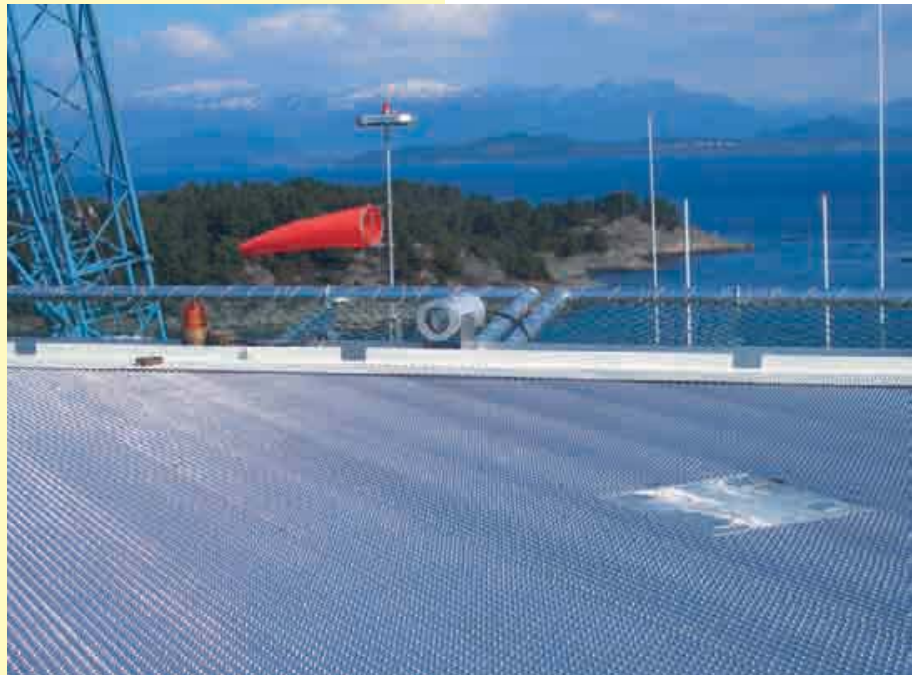
Figure 1: Helideck with explosion protected floodlights and perimeter lights of Tranberg
