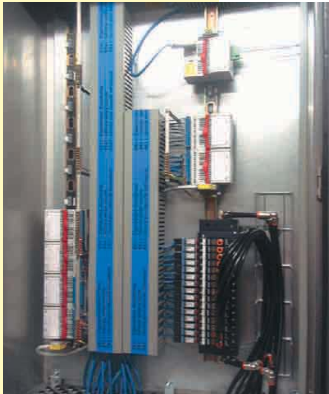
Figure 1: Remote I/O system with control valves fitted
