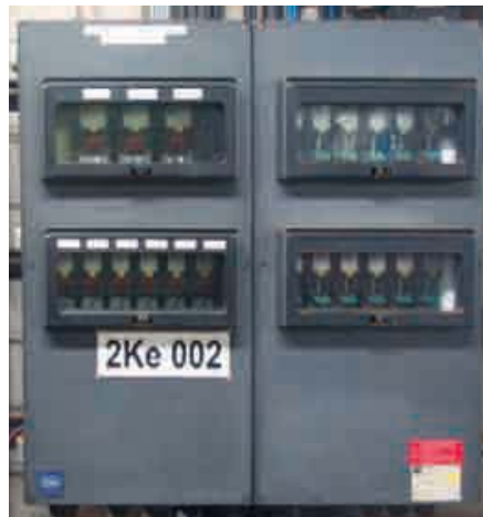
Figure 3: Miniature circuit breaker distribution boards with housings in »increased safety« and circuit breakers in »flameproof enclosure« are operated from the outside via flaps
