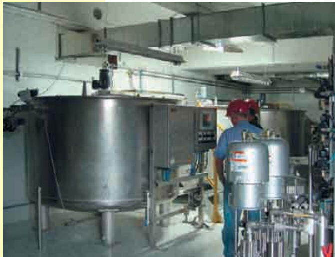
Figure 1: Paint conditioning station in the paint mixing plant during commissioning without the presence of an explosive atmosphere
