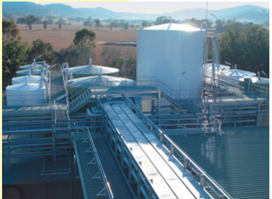
Figure 1: Production plant for Bio-Diesel fuel
