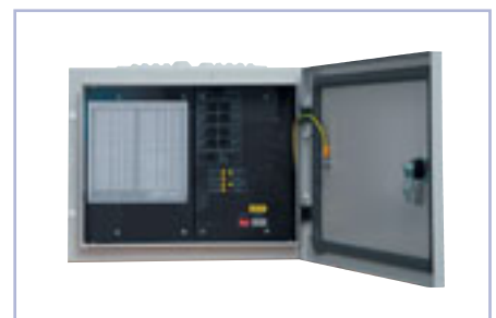
Figure 6: Miniature sub-station in E30 enclosure
