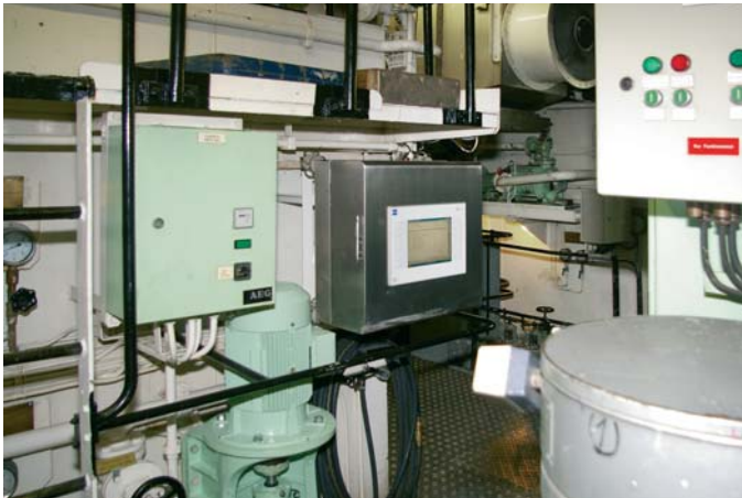
Figure 2: The explosion protected HMI in the engine room supports the data communication network and makes for a more user-friendly operation
